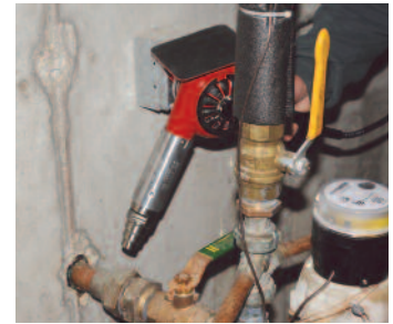
Heat pipes and more
